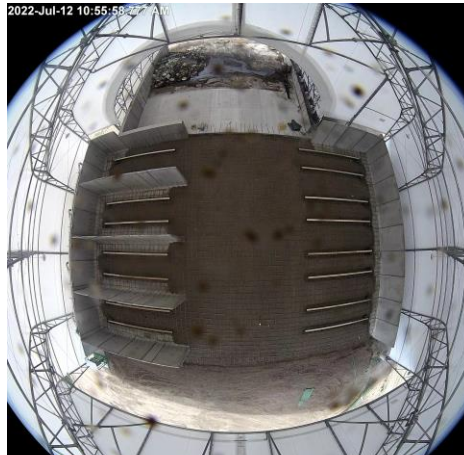
GRCF aerial snapshot of the tipping floor (top) and the bunker/aeration areas (bottom) before concrete was poured, showing the aeration piping embedded in the floor.
